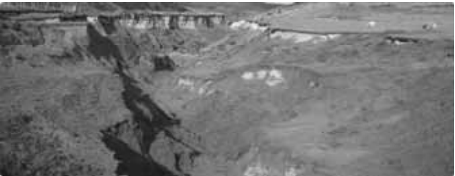
Plate 23: Localised gully erosion in unconsolidated sands. Caused by ineffective management of a water overflow (MT).
