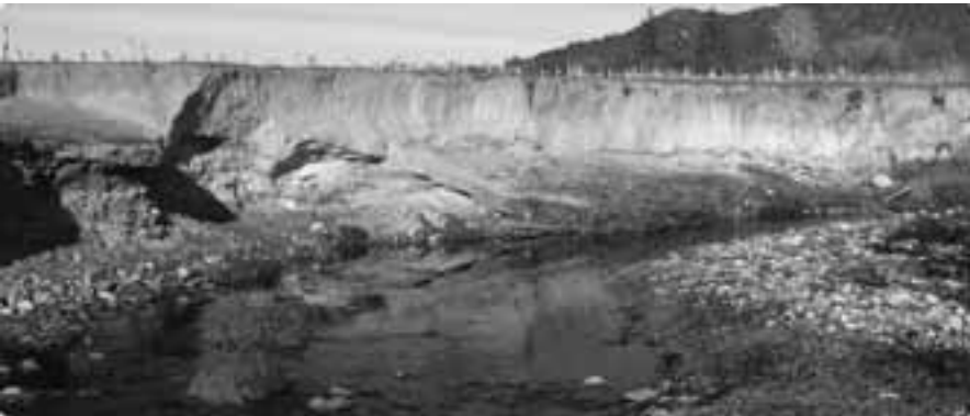
Plate 29: Severe streambank erosion of fine-grained alluvial soils overlying weathered alluvial valley fill gravels of the Sherry catchment in the Nelson region (TDC).
