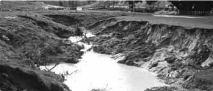
Plate 28: Moderate streambank erosion south of Tinui, Wairarapa (MJP).
